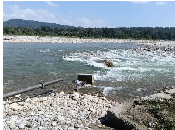
Image 7-4: Damaged sewer line between Pampapuri to Fooltal I&D
