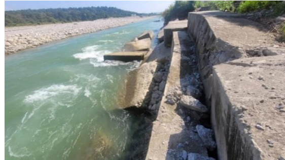
Image 7-1: Sliding and overturning of concrete blocks due to scouring
